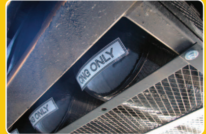
Five CNG tanks (65 diesel gallon equivalent).
